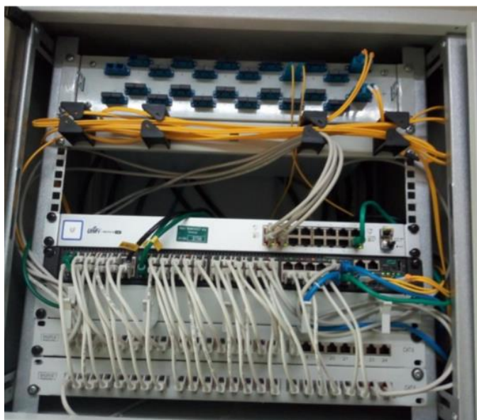
Figure 5. Example of a network cabinet with equipment at a remote location Bešin - Old Administration
